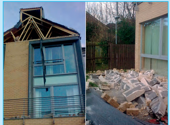
Storm damage to residential housing in Burnside, South Lanarkshire
