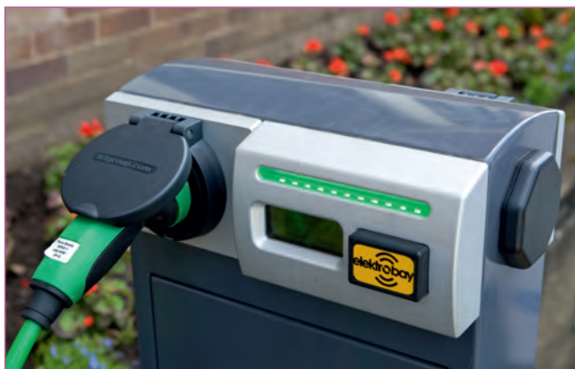
Electric charging points
