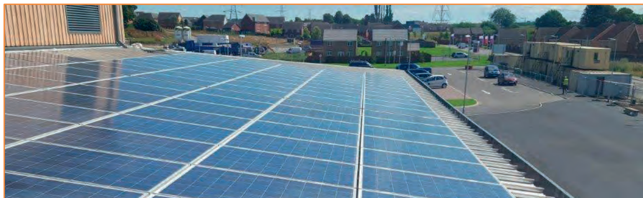
Solar panels at Newton Farm Primary School, South Lanarkshire
